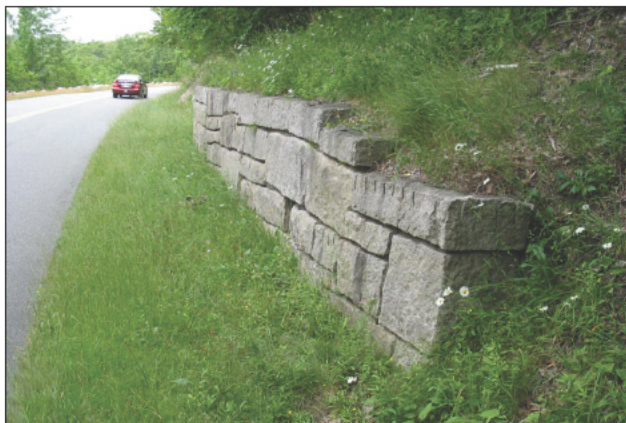
Figure 19-misc1. Looking north at the retaining wall associated with the Vista 19 centerline (OCLP, Acad0012_1.879, 2005).
